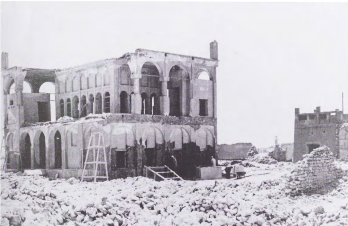
(Fig. 8) : The Center Majlis and the Eastern flank of the Sheikh Abdullah's residence under restoration.
